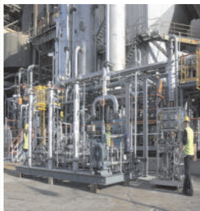
PVSA Demo plant at Hazelwood Power Plant, Australia
