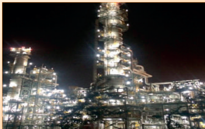
The Benzene Recovery unit (BRU) by night
