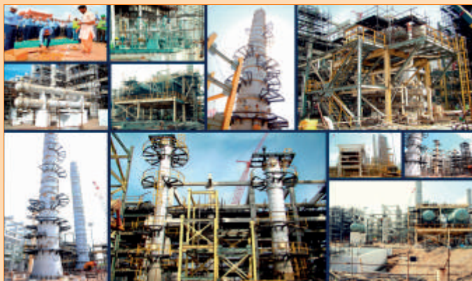
Civil / Construction Work of the Benzene Recovery Unit at RIL Jamnagar (circa late December, 2014)
